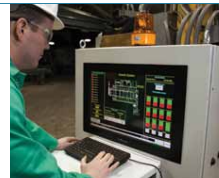
Line central controller monitors and controls all manufacturing process parameters.
